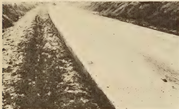
FIGURE 4.—SHOULDERS ARE RUTTED TO A DEPTH OF 4 INCHES BELOW BOTTOM OF SLAB
